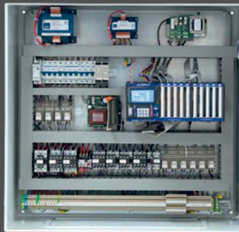
Hydraulic Control Panel
